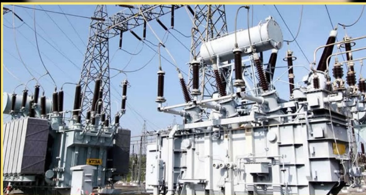
This image shows a KTBA power transformer in a substation, which is a critical piece of infrastructure for electrical grid management. Photo credits; The Guardian Nigerian News
